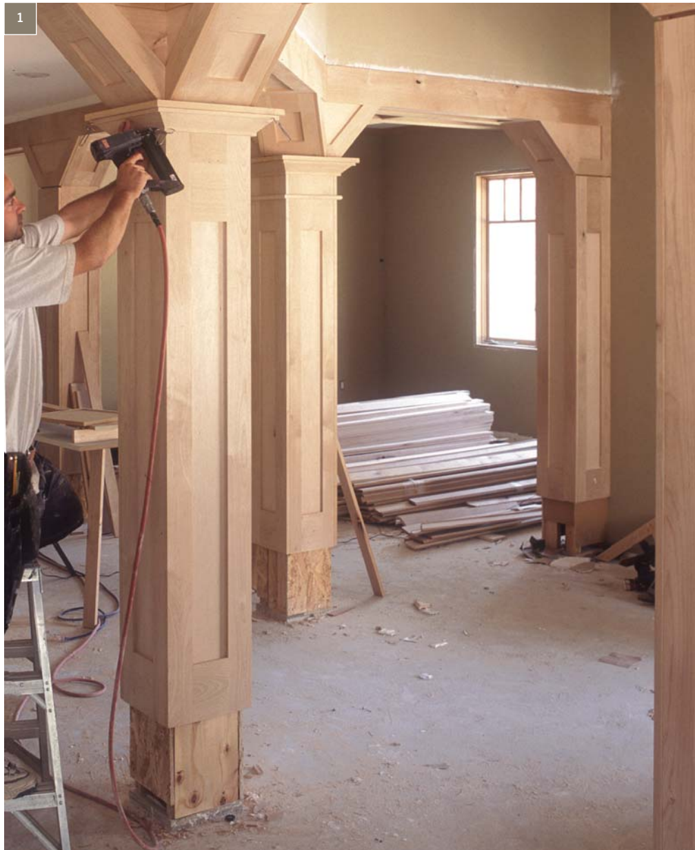
FIG. 1: I've always stored trim material right on the wood subfloor, or on 2x4 sticking when I'm working on a concrete slab. At night, I was taught to cover my trim material with a tarp.
